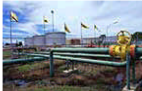
B26- OIL PLANT
